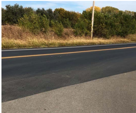
This picture shows an area on Radio Lane that was recently coated with the HA-5 Sealant.
